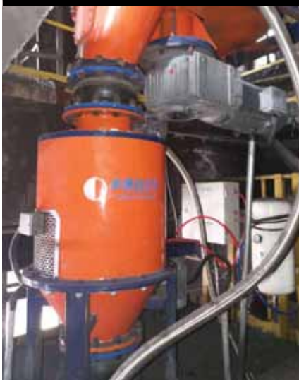
Application of a Coriolis pulverised coal feeder
